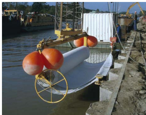
Figure 4: GCL and sand mat separately enrolled on a spreader bar as lining system for underwater installation (Fleischer & Heibaum, 2002)
