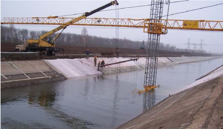
Figure 5: Underwater installation of the sand mat and GCL composite in a drinking water canal in the Ukraine, 2004
