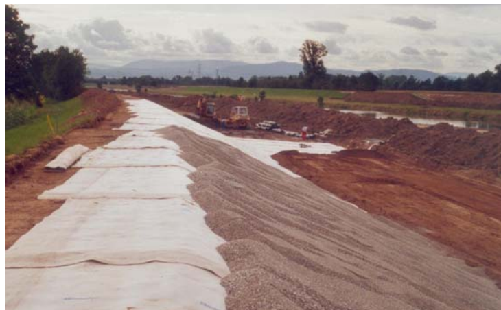
Figure 8: Rehabilitation of the Kinzig river levee in 2001 with GCL - installation of non-cohesive river gravel as cover soil for the GCL (Heerten et al., 2008)
