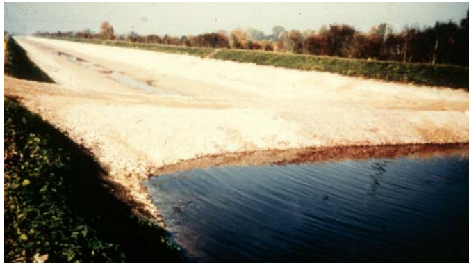
Figure 1: Rehabilitation of the hydropower canal Lech in 1989 – easy coffer dam lining with GCL
