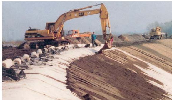
Fig. 4 Lippe River levee reconstruction (1994): Installing Bentofix® GCL as a levee seal (Saathoff & Werth 2003)
