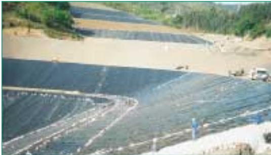
Figure 3 Carbofol® and Bentofix® composite liner in a municipal landfill (landfill Argalarío, Spain).
