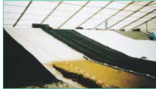
Figure 24 Installed Carbofol®/ Bentofix®/Secudrän® composite sealing system on a contaminated sand dam (noise barrier Hohenbudberg, Germany).
