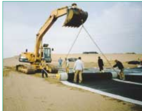
1995, landfill caps were sealed with Carbofol® geomembranes and Bentofix® geosynthetic clay liners.
