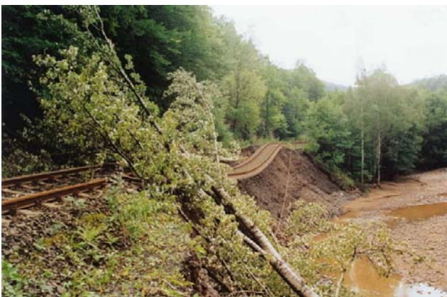
Fig. 18: Collapsed railway embankment after flooding
