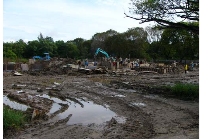
Fig. 17: Limited rutting of reinforced base courses
