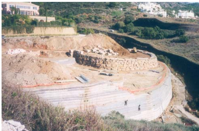
Fig. 24: Installation of natural stone block facing for the semi-circled geogrid reinforced soil structure (August 2003)
