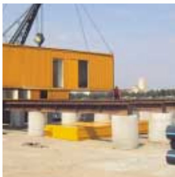
Geobarrier® flood protection by elevating a container park with Combigrid® in Rheinau Harbour, Cologne, Germany
