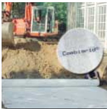
Combigrid® in action beneath the base course of the bus terminal in Melle-Wellingholzhausen, Germany
