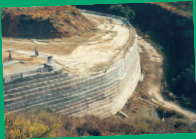
Fig. 4 Installation of natural rock blocks as facing for the geogrid reinforced soil structure
