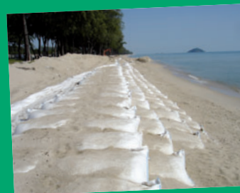
Fig. 7 Terrafix Soft Rock® protected beach line while being covered with beach sand
