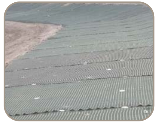
The use of the ArmorMax® System allowed the project to proceed quickly and efficiently.
