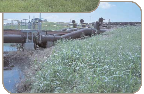
September 2008: ArmorMax™ protected slope after Hurricane Gustav.
